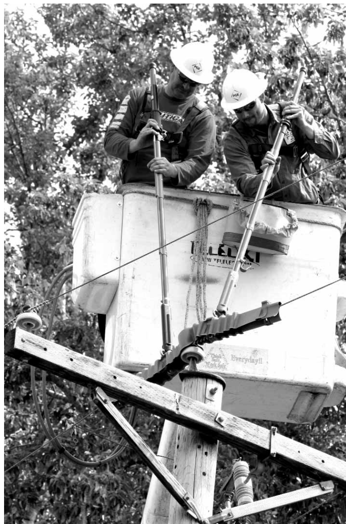
PGE linemen install wire covers and anti-perching devices along Reeder Road on Sauvie Island.
