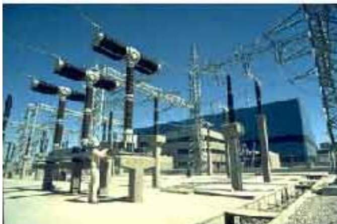
Transmission Substation: Controls the transmission of electricity into a high-voltage network from a power plant.
