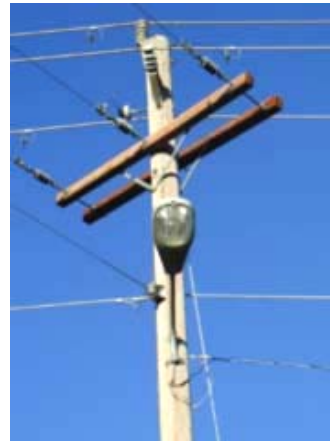
Power Poles: Carries lower voltage electricity from substations to houses.
