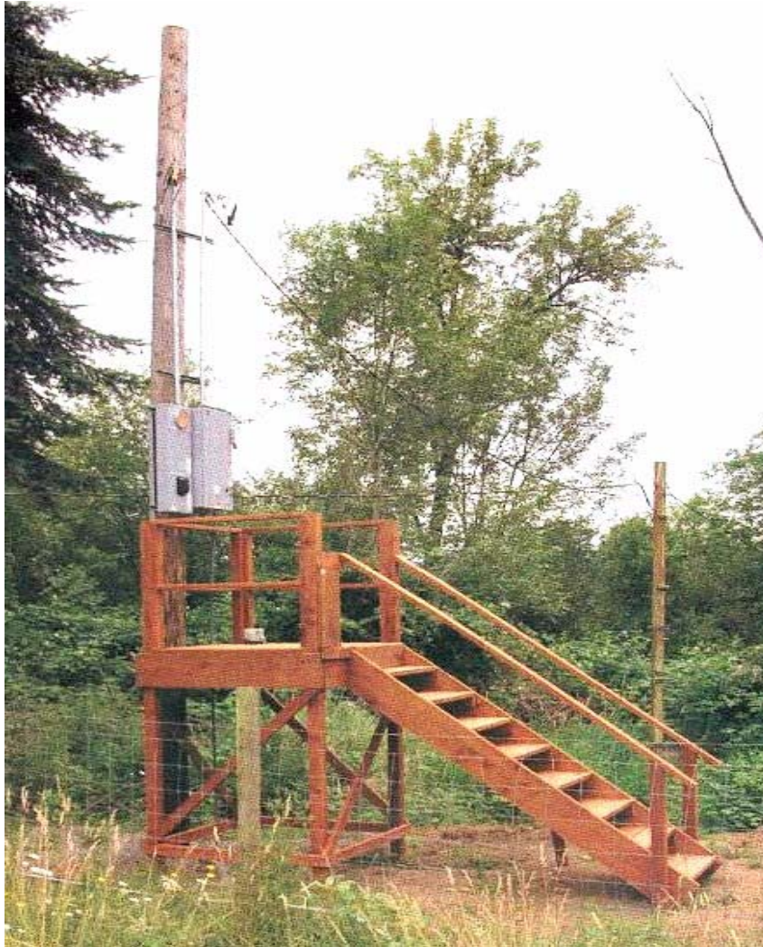
Figure 12-4 Customer Built Platform
